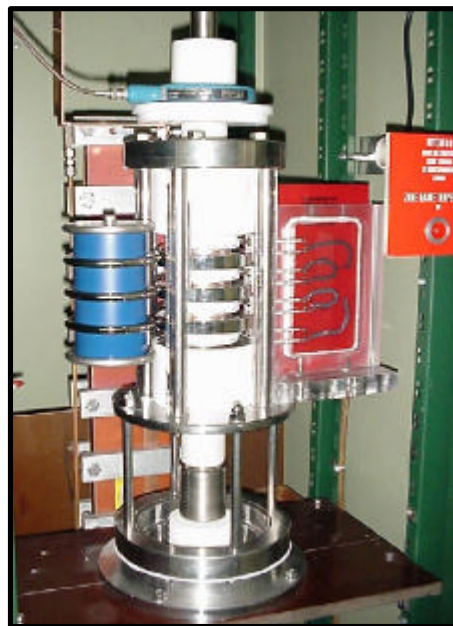
Fig. 3: Installed MKDH switch
